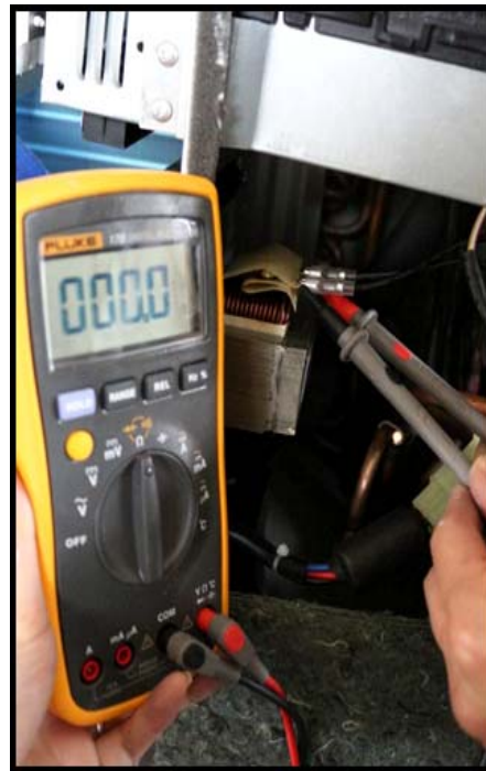
Fig. 24 – Test the Reactor Resistance
