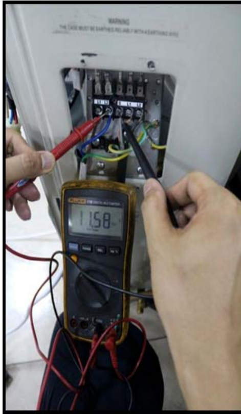
Fig. 23 – Test the DC Voltage
