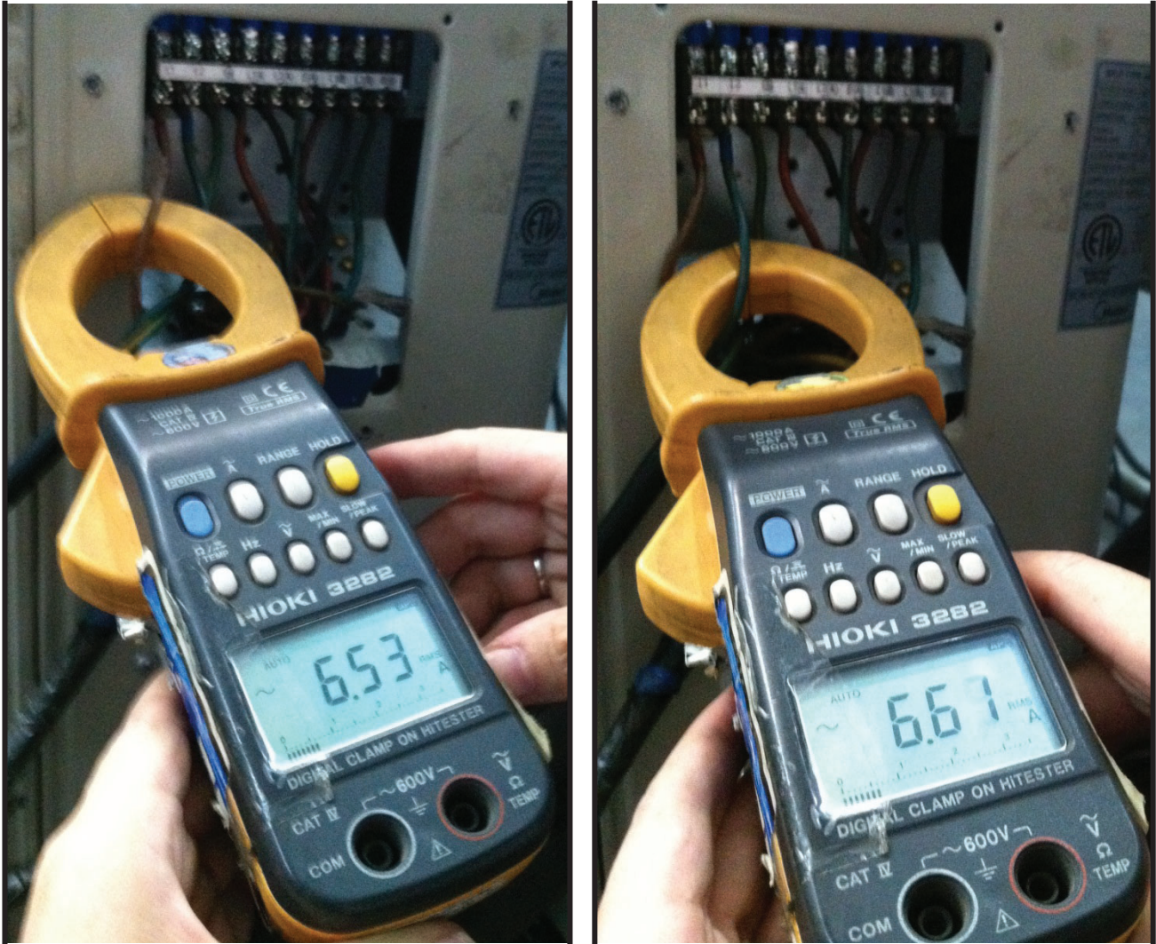
Fig. 62 – Test the amperage
