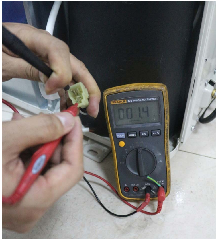
Fig. 63 – Test the voltage
