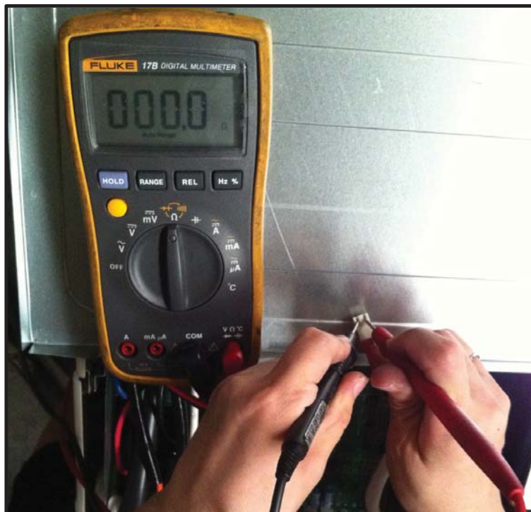
Fig. 58 – Test the voltage
