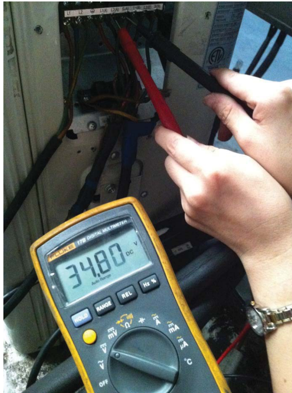
Fig. 41 – Test the DC voltage
